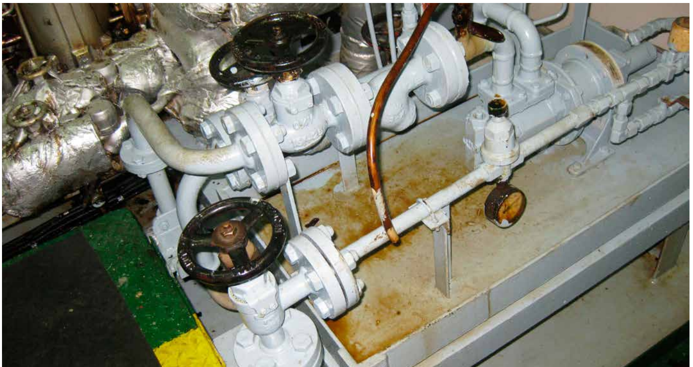
Poor sampling location: not on the main line and not a clean pipe with shape edge to prevent dirt build-up
