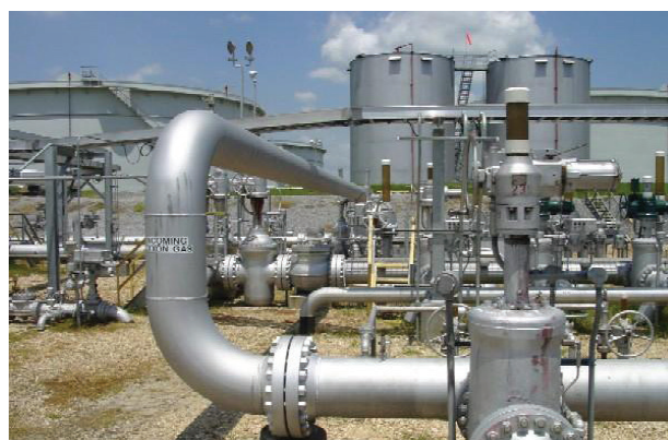
Shore pipelines and valves
