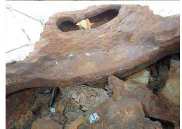
A container foundation's very poor condition makes it unserviceable
